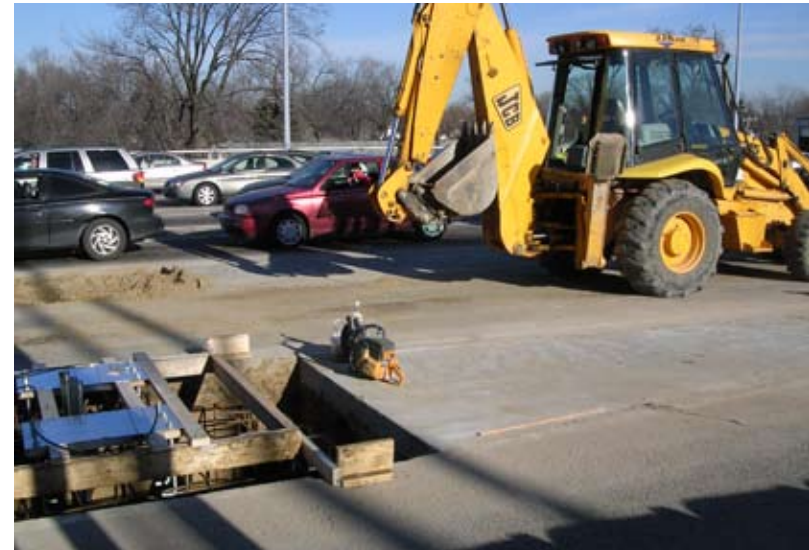
Infrastructure needs and construction projects are included in CBP and GSA capital programs each year.
